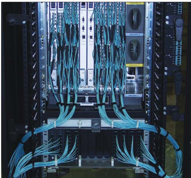
Figure 20: Cabling Various Director Blades with U-Space System
