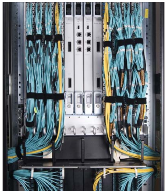
Figure 2: 384-Port DCX with Corning Cable Systems Cabling Solution
